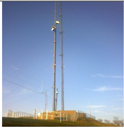
EMS Transmitter Site
