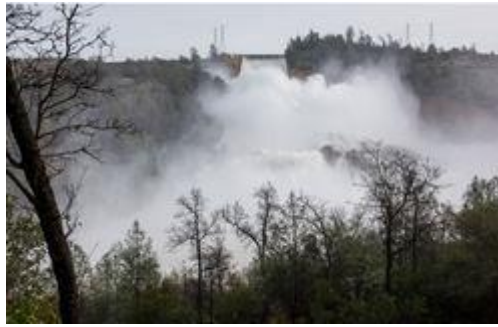
The California Department of Water Resources released 100,000 cubic feet per second from the damaged spillway to decrease the lake level by 50 feet to handle the next round of storms expected this week. [California DWR photo by Kelly M. Grow]
