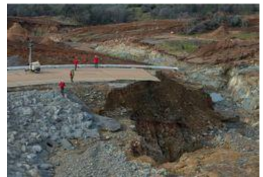
California Department of Water Resources crews inspect and evaluate the erosion just below the Lake Oroville emergency spillway site after lake levels receded on February 13. [California DWR photo by Kelly M. Grow]
